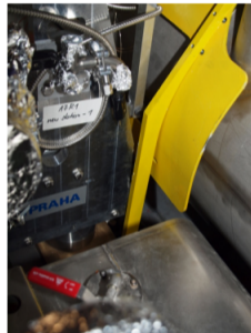
QRL-protection very close to station
